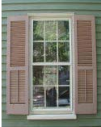
Storm window properly installed
